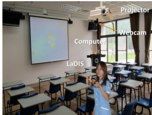
Figure 1(b). Set-up of a real system: (1) the webcam can be fixed on a projector (2) the projector usually hangs from the ceiling of classroom (3) the computer usually is set up inside a lectern (4) wireless control technology can connect with LaDIS and a computer without any connecting lines
